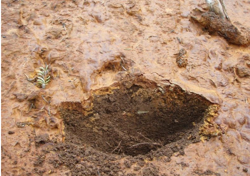
Figure 77. Formation of iron ferricrete from AMD water.
