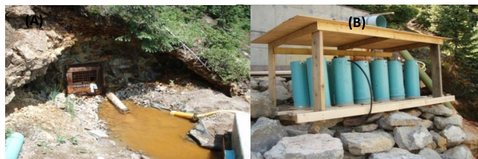
Figure 38. Eveline mine draining adit (A) and treatment columns (B)
